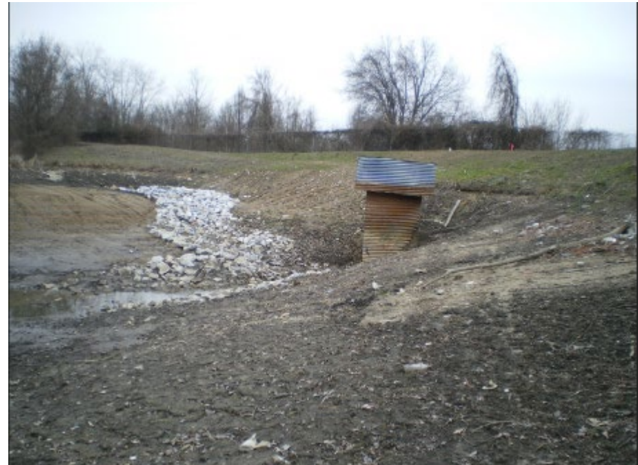
Riser Structure Corrosion
