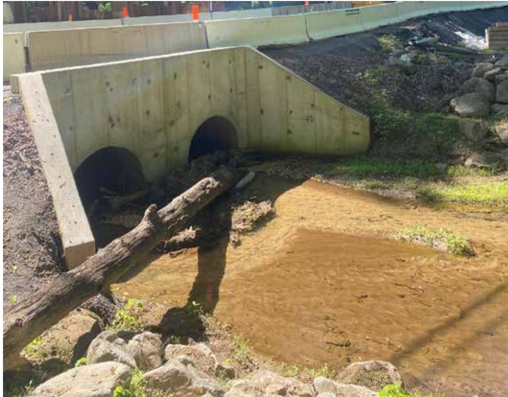
January 2021 –Twin 60" RCP with Headwall
