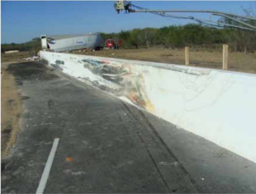
Fig. 11. General view of the barrier wall after vehicle impact
