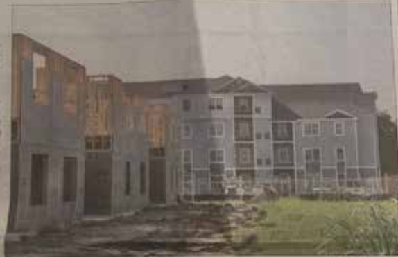
Affordable-priced apartments are under construction on Elliott Road. Easton's housing task force met last week to prioritize which housing recommendations it should make to council members as the town aims to address its shortage of affordable housing.
